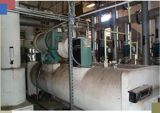
An air conditioning chiller is a heat exchanger that cools down water. The water is circulated through the building to various cooling coils located in ductwork.
